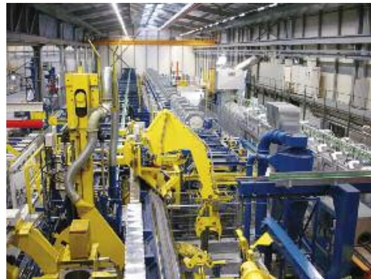
The Dornach plant is equipped with a modern foundry and continuous extrusion, pressing, rolling and drawing machinery
